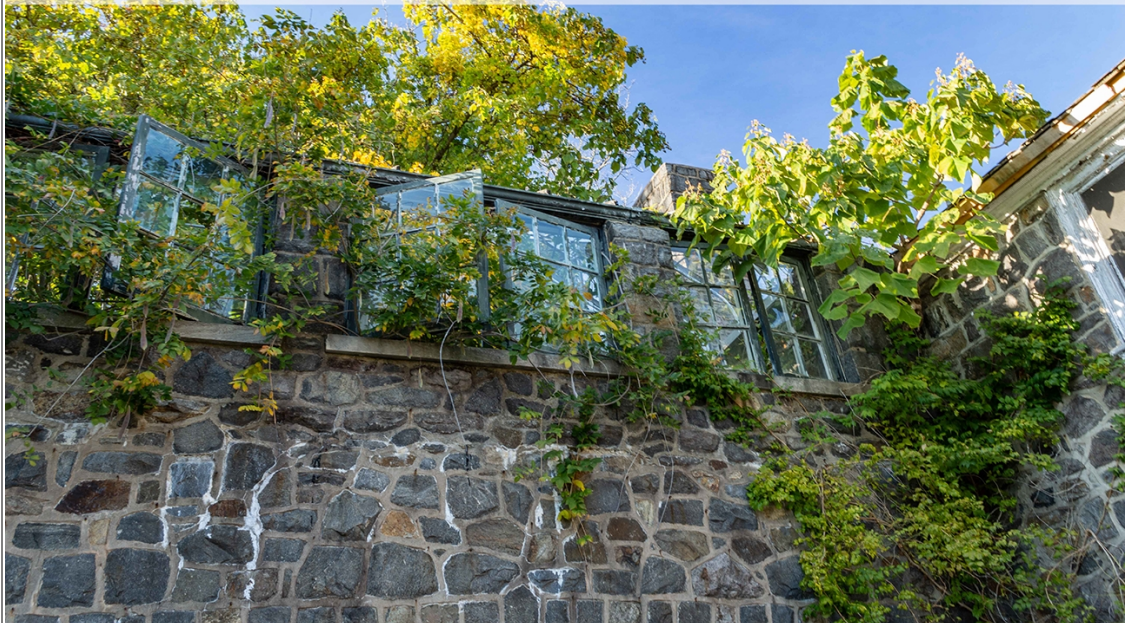
Gibraltar- Greenhouse 11 06 2021 Missing & Open Windows; Open Roof
