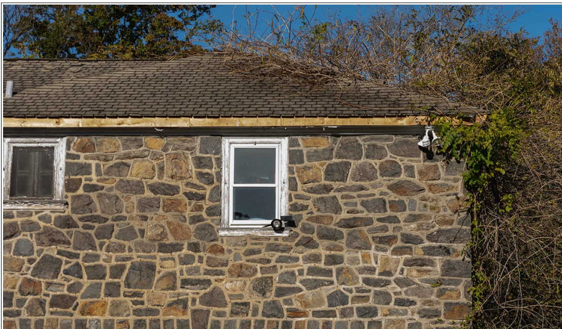
Gibraltar- Garage & Chauffers' Apartment Southern Facade 11 06 2021 Missing Gutter, Vines overtaking building and roof; new window
