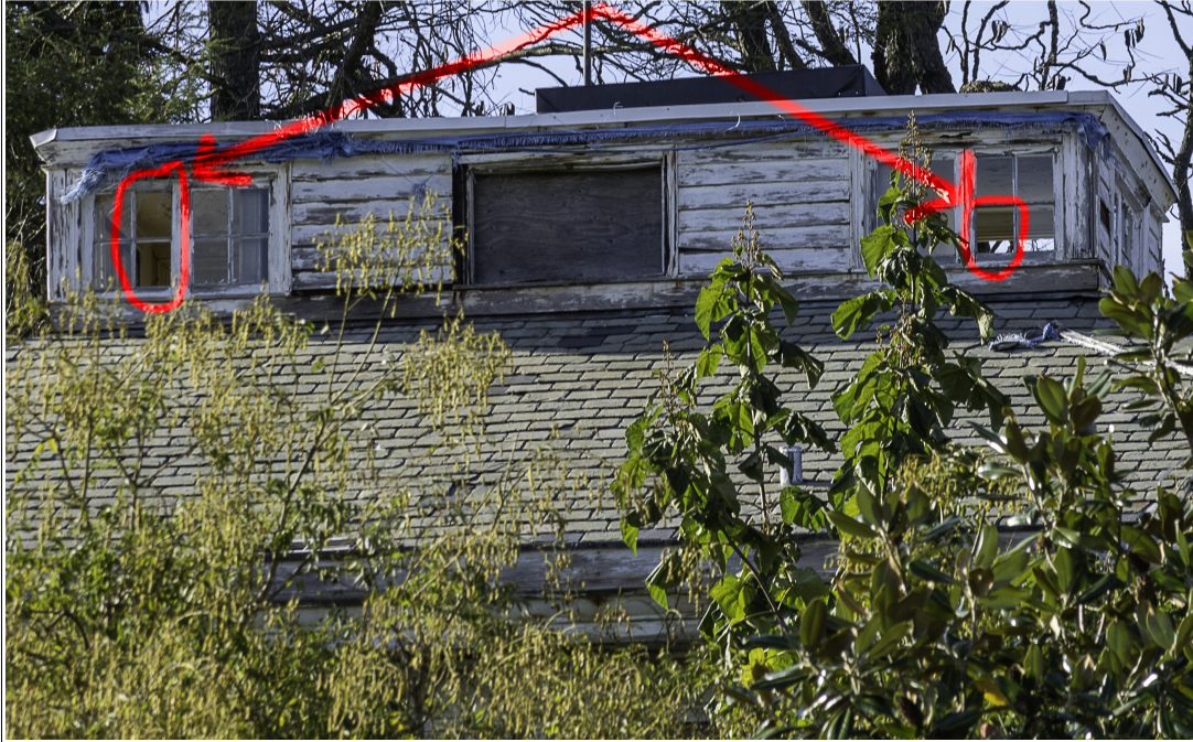
Gibraltar – Mansion Eastern Facade - 11 06 2021 Missing Window Panes
