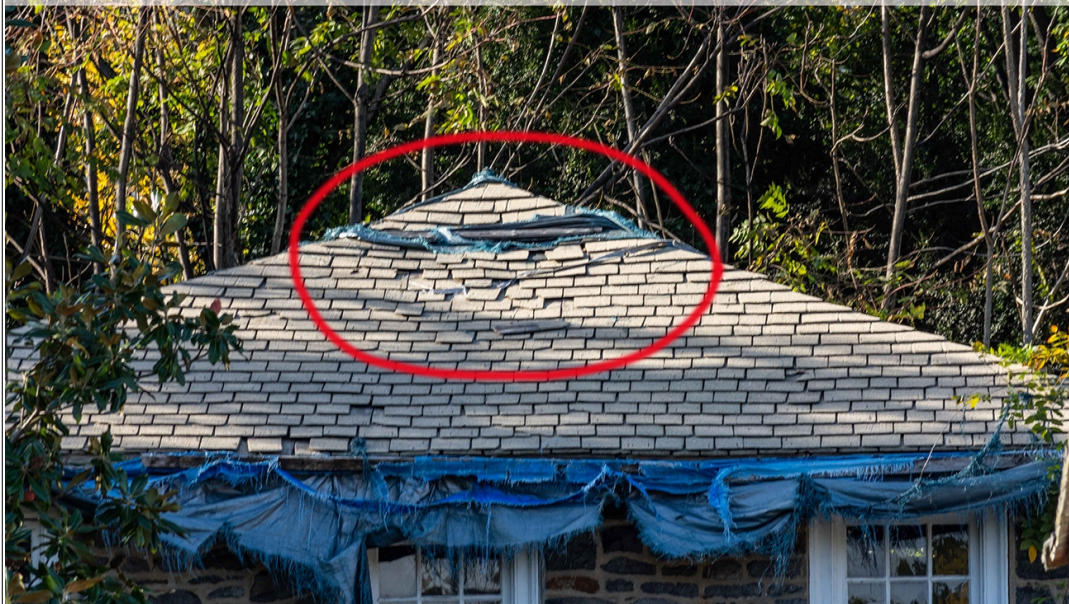
Gibraltar- Pool House Eastern Facade #2 11 06 2021 Roof beginning to collapse
