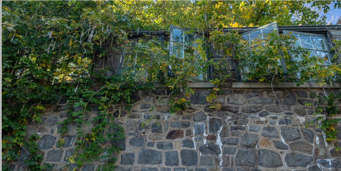
Gibraltar- Greenhouse - Southern Facade 11 06 2021 Open roof; Missing & Open Windows Vines, Weeds & Trees
